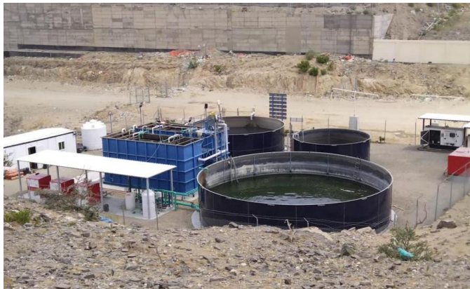
Figure 1: Membrane Bio Reactor (MBR) plant
