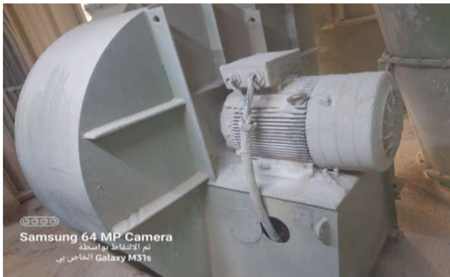
Figure 9: A Typical High-Pressure Fan used in Atbara Flour Mill Factories
