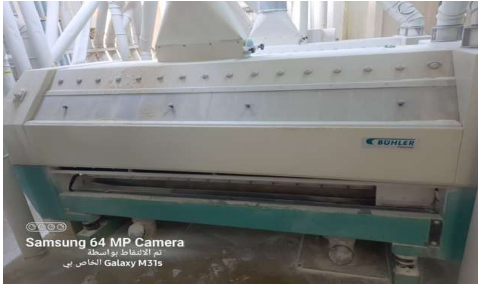
Figure 8: A Typical Semolina Sieve used in Atbara Flour Mill Factories
