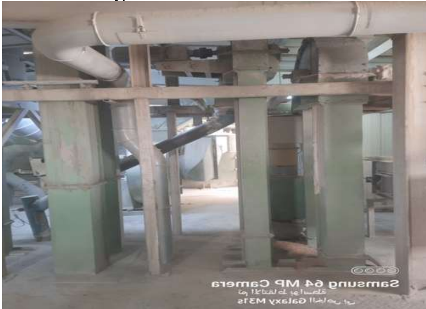
Figure 4: A Typical Bucket Elevator used in Atbara Flour Mill Factories
