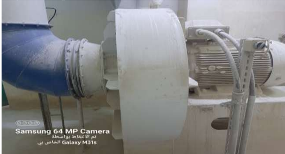
Figure 10: A Typical Low-Pressure Fan used in Atbara Flour Mill Factories
